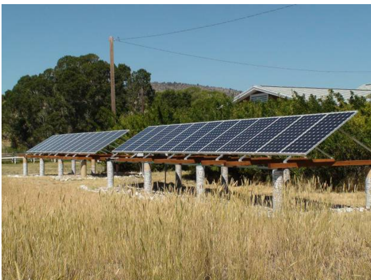
Madison Ranger Station PV installation
