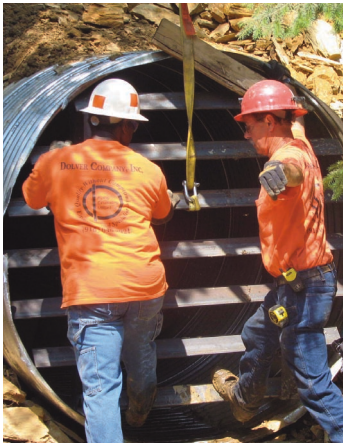
Closing an abandoned mine and installing a bat access screen was a partnership between the Office of Mine Reclamation and the Forest Service.
