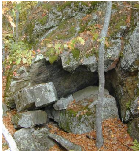
Old mine shaft, where gaping hole was filled by blasting surrounding rock and causing a rock fall
