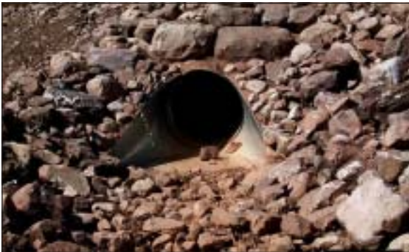
Oversized culverts on steep gradient channels allow passage of large channel substrate rocks.
