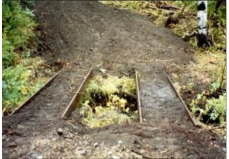
Temporary bridging methods allow for heavy equipment to cross streams with minimal disturbance to channels.
