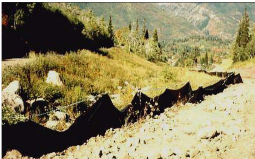
Vegetation buffer strips should vary in width based upon side-slope gradient. Where only a narrow strip is present, it should be supplemented with other sediment control practices such as silt fences or straw bale dikes.
