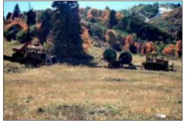
Direct burial of electrical lines reduces the width of utility corridor disturbance when compared to trackhoe excavated trenching.
