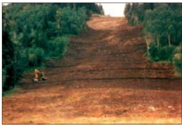
A trackhoe excavator can quickly construct a very effective waterbar drainage network on steep ski runs.
