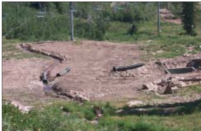
This stream has been moved away from new impacts and into the original channel that existed before the chairlift and ski run were constructed.
