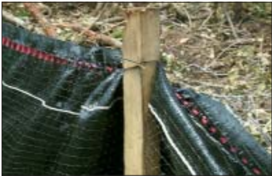
Deep snow will strip a silt fence from its support stakes. Securing the fabric to the stake with cable ties or wire prevents this.
