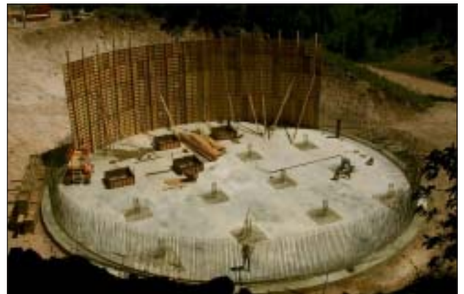
Storage tanks must be cleaned of contaminants before use. This can generate waste water that should be treated prior to discharge.
