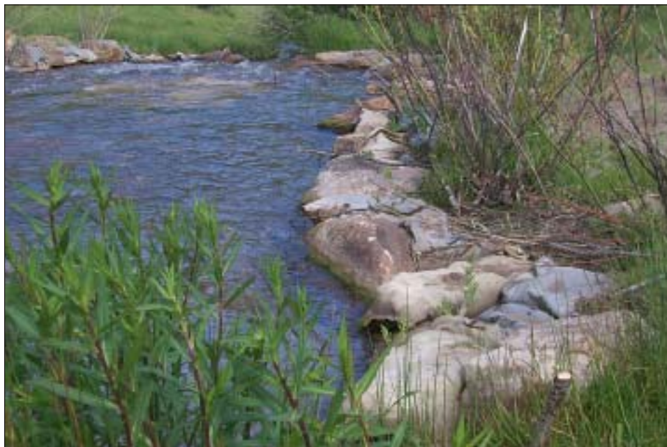
Armored channels can be revegetated with burlap bag "soil pillows" and with willow soil-root plugs.
