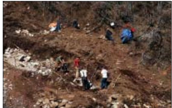
Tower foundations in steep or remote terrain may require excavation by hand crews.
