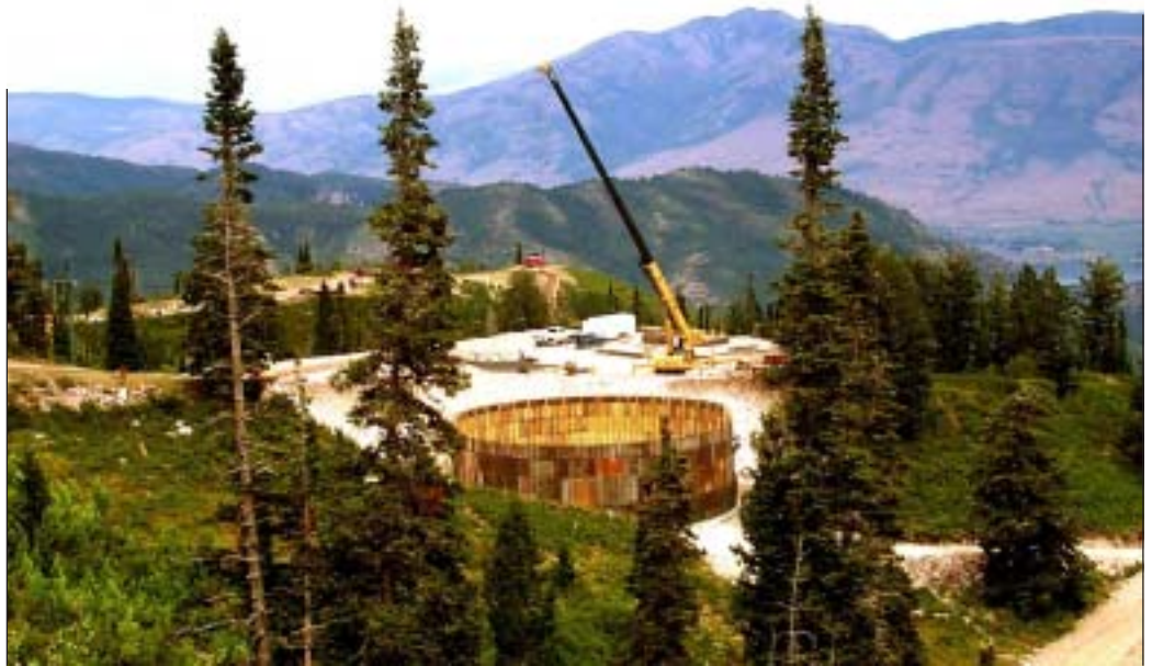
Staging areas and access roads can be built from storage tank excavation material.
