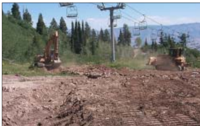
Small trackhoes and bulldozers provide a lighter touch and are better suited to the fine detail work needed in stream reclamation.
