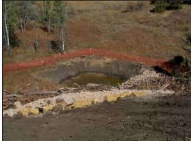
Runoff from large cut or fill slopes should be routed through sediment trap basins.
