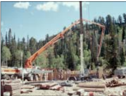
Staging areas for construction projects can be a significant source for fuel/oil, cement, and sediment pollution to adjacent streams.
