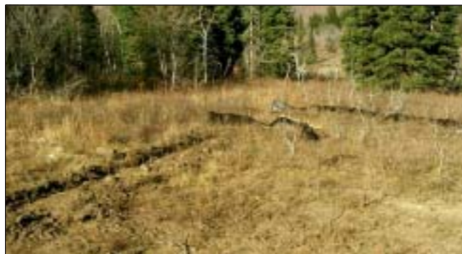
Discharge water from detention basins can be routed through straw bales and silt fence for more complete sediment removal.
