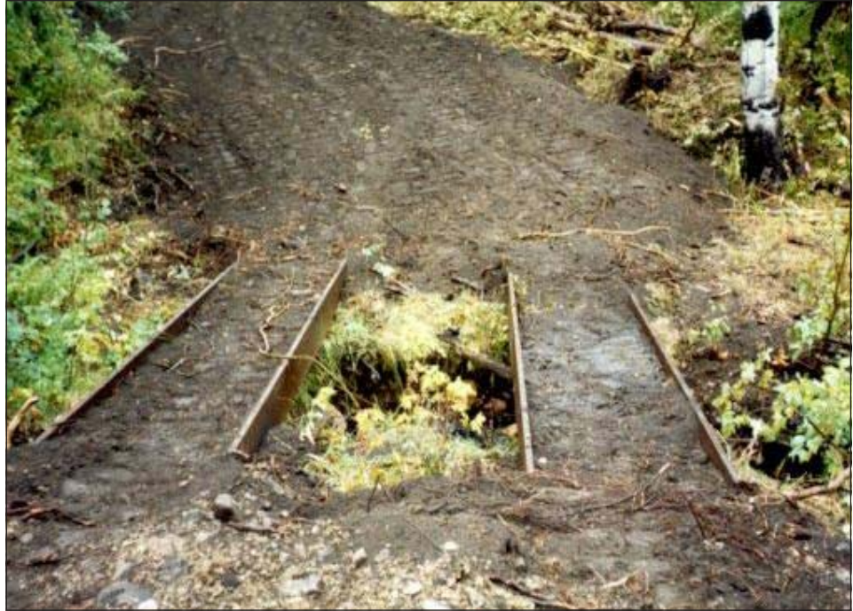
Steel "I" beams can provide effective and low cost access for heavy equipment across streams with minimal channel damage.
