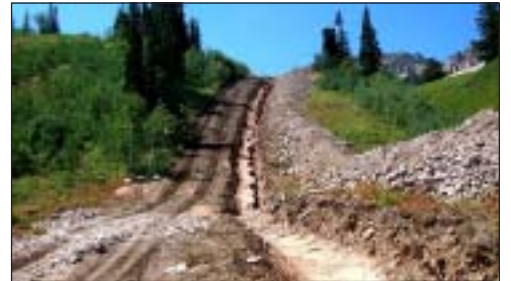
Pipeline trenches, can quickly turn into stream channels if not protected from rainstorm runoff.
