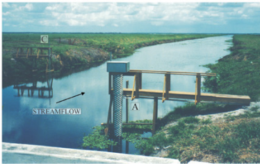
TYPICAL ACOUSTIC VELOCITY METER SITE
