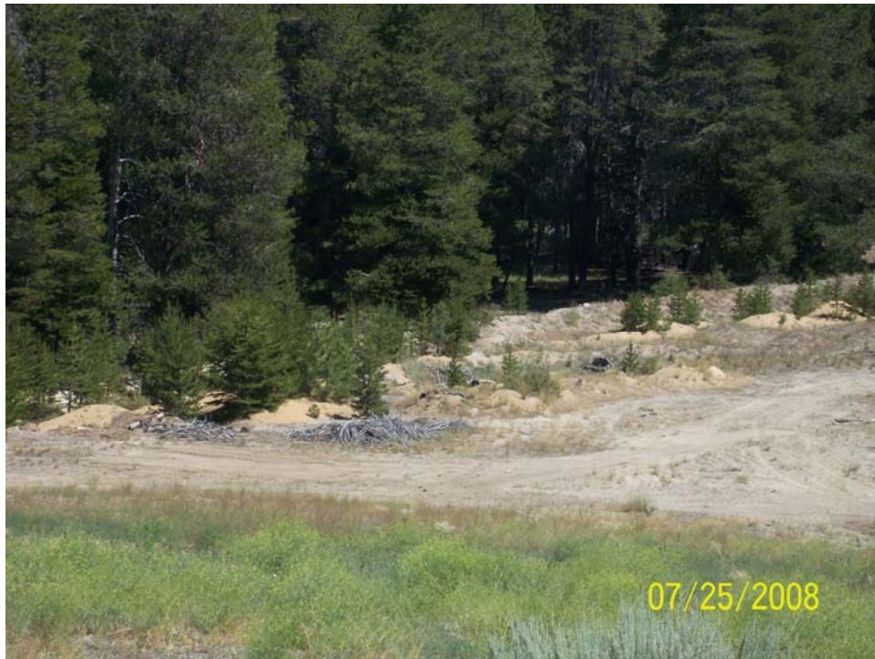
Photograph A-16. USFS – Meyers Landfill: – ML-TP-03 PERC-1 backfilled and restored. Photographed: July 25, 2008
