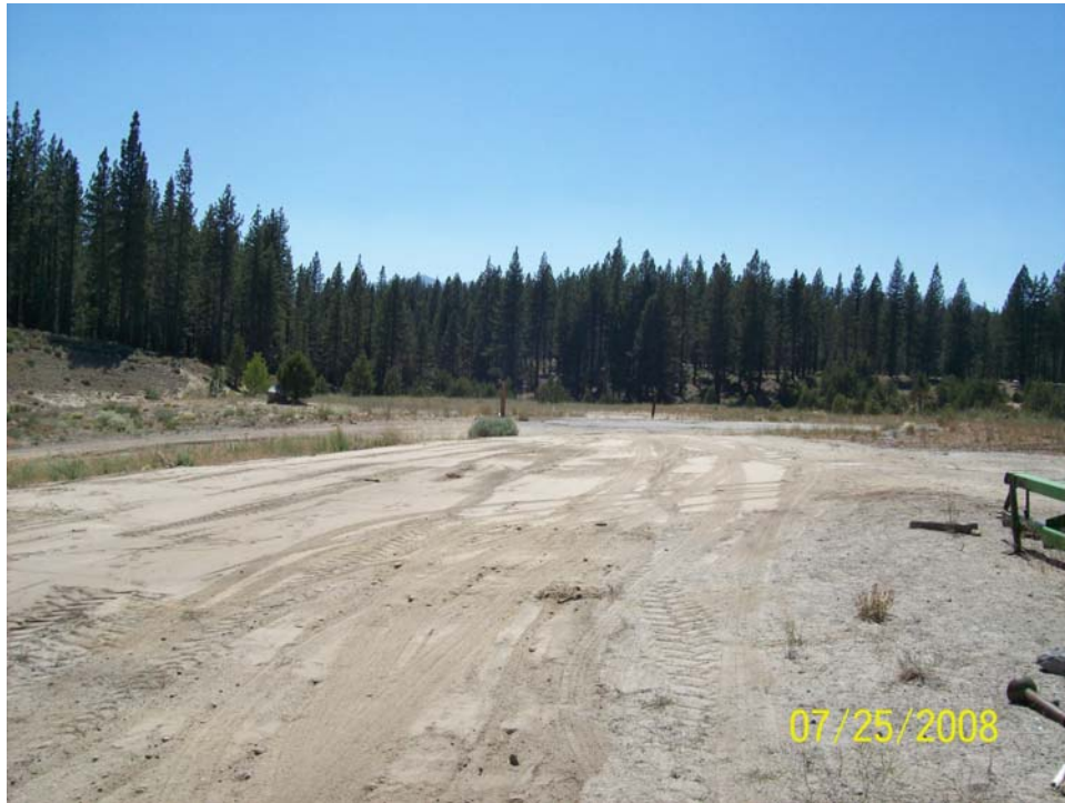
Photograph A-15. USFS – Meyers Landfill – ML-TP-02 and ML-TP-02 PERC-1 backfilled and restored. Photographed: July 25, 2008
