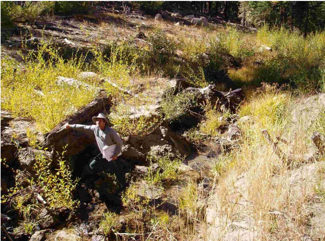
Photo 8. Significant bank erosion has occurred at pp 3a, Oct. 12, 2006.
