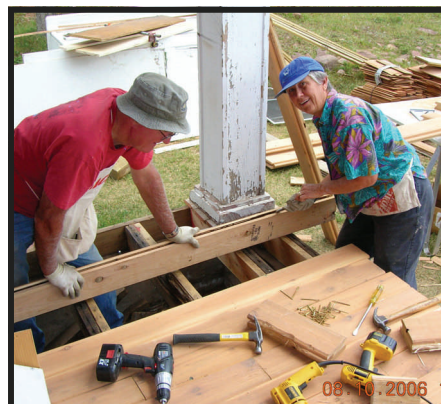
Ashley National Forest Recreation and Heritage Crews worked together with Volunteers to replace the Cabin's porch/deck and renovate the kitchen.
