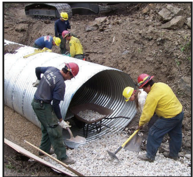
Lots of rock to move at the upper Gance Creek site. Fire crew helps the fish biologist (yellow hard-hat, center) fill the culvert.
