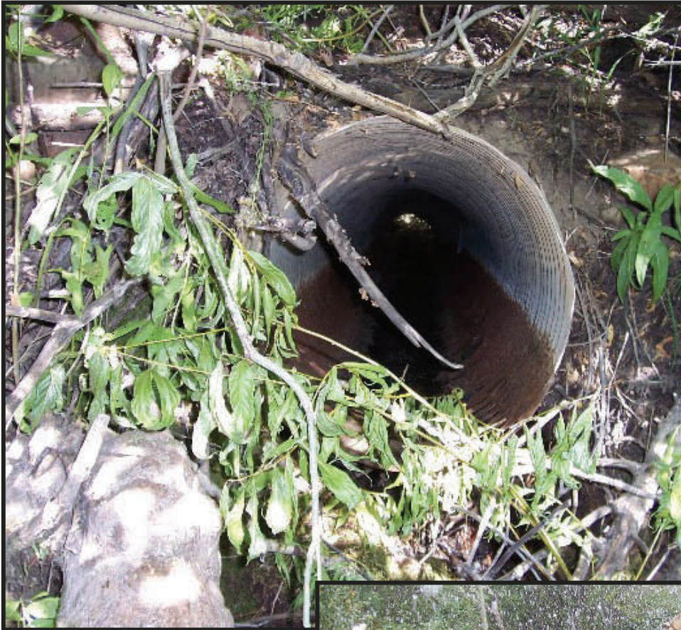
Upper Gance Creek crossing. Preimplementation. Looking upstream at culvert (24" diameter). Brush obscures a perched condition 18+".
