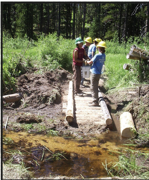
Students from the Student Conservation Corps worked hard to complete a turnpike structure and install a curb along the Phoebe Meadows Trail.
