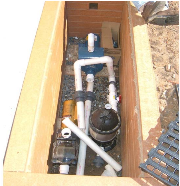
“Green” equipment bunker
