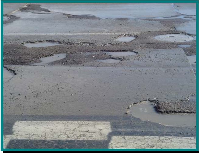
Pavement requiring rehabilitation or reconstruction.
