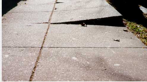
Figure 4-36. Changes of level in sidewalks caused by tree roots are potentially hazardous for pedestrians.
