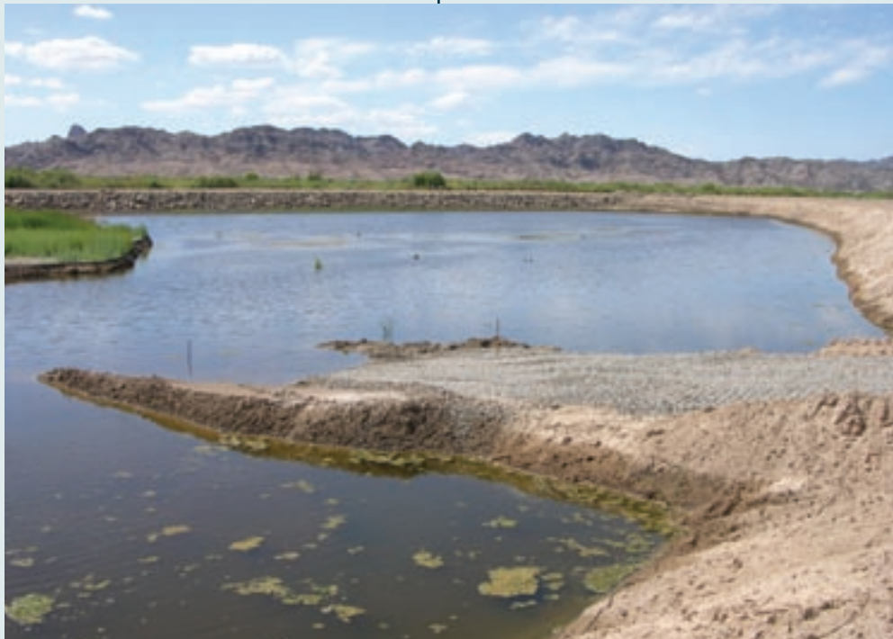
Six new ponds are being excavated at Imperial National Wildlife Refuge in Arizona as part of the Lower Colorado Multi-Species Conservation Plan. The ponds will provide new habitat for two endangered fish – the razorback sucker and bonytail. (USFWS)
