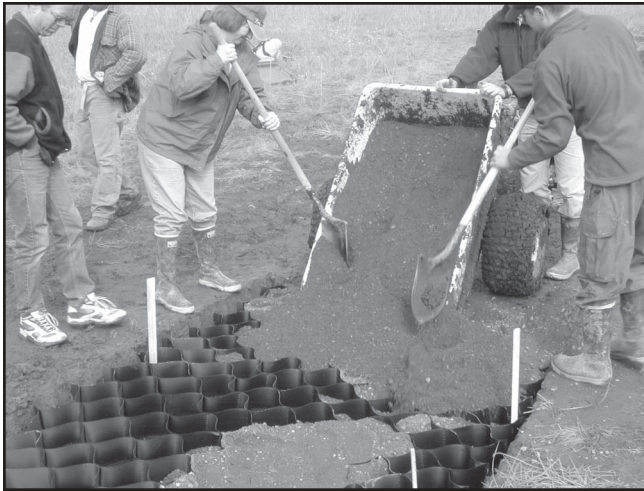
Figure 13—A cellular confinement system being installed on an experimental trail in southcentral Alaska. Four-inch-deep cells were formed by expanding the cellular product accordion style, then backfilling and compacting with a suitable fill material—in this case, sandy gravel. The sides of the installation were confined by a 6-inch-deep trench.
