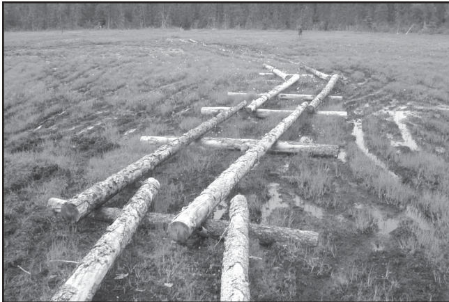
Figure 19—Rough layout of the sill and stringer timbers for puncheon trail construction over a wetland area in southcentral Alaska. Stringers are laid with tops meeting tops and butts meeting butts.
