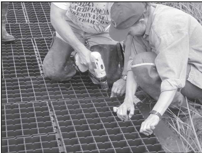
Figure B7—Joining the sections using a screw gun. Note the underlying plywood.
