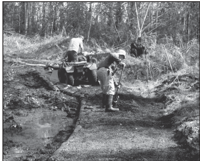
Figure 12—A geotextile and gravel-cap installation over permafrost-degraded soils in Yukon-Charley Rivers National Preserve in Alaska. Use of geotextile and a gravel cap on this trail allowed the National Park Service to construct a 6-foot-wide OHV trail over a 3- to 4-foot-deep muck hole.
