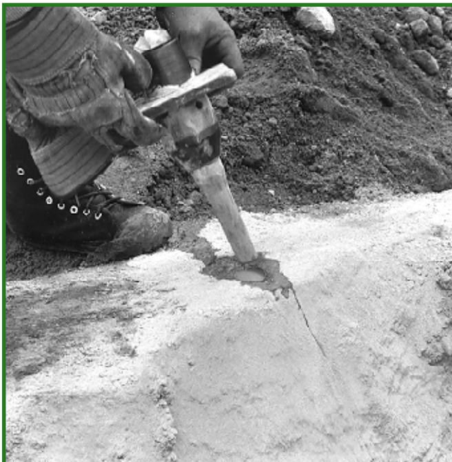
Figure 5—The impulse barrel and breech block assembly is placed in the hole.
