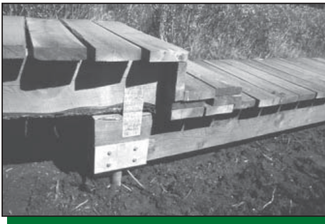
Figure 38—A helical pile was used for this boardwalk. Stringers are attached directly to the beam saddle, helping to keep the boardwalk close to the ground.
