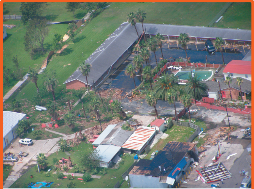
Figure 1. Hurricane Humberto caused wind damage to a Food Mart/ Gas Station on High Island. Note the awning collapse at a gas station in the lower right, wooden debris in the center and fences blown down in the upper left. Photo is courtesy of the Galveston County Office of Emergency Management.
