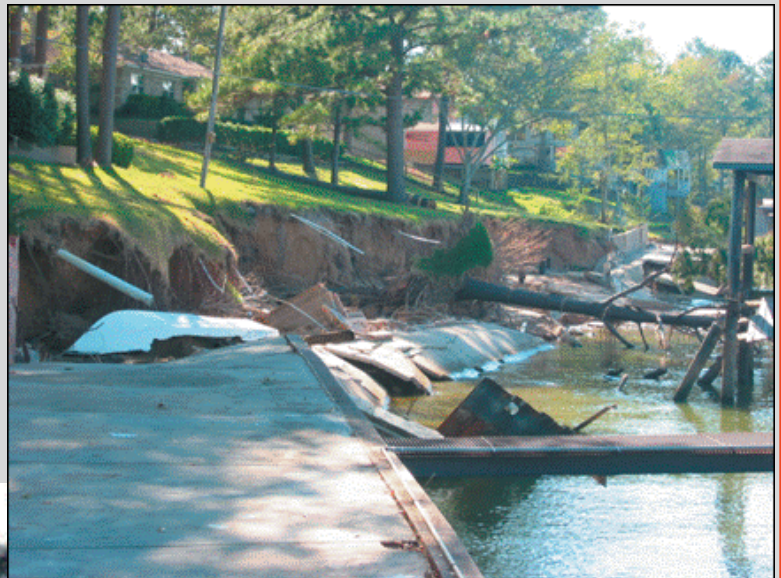
Figure 4. Damage to lake front lots at the point of the Indian Hills subdivision.
