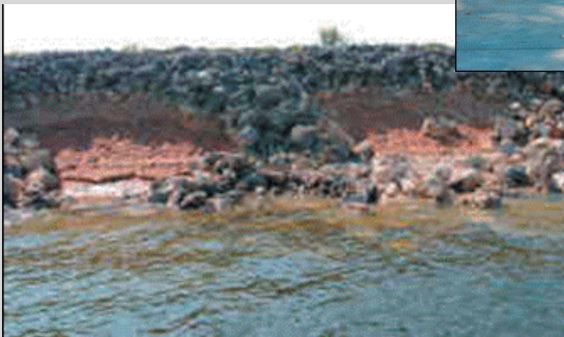
Figure 5. Erosion to the Lake Conroe Dam east of the main gates. Image from Montgomery County News.
