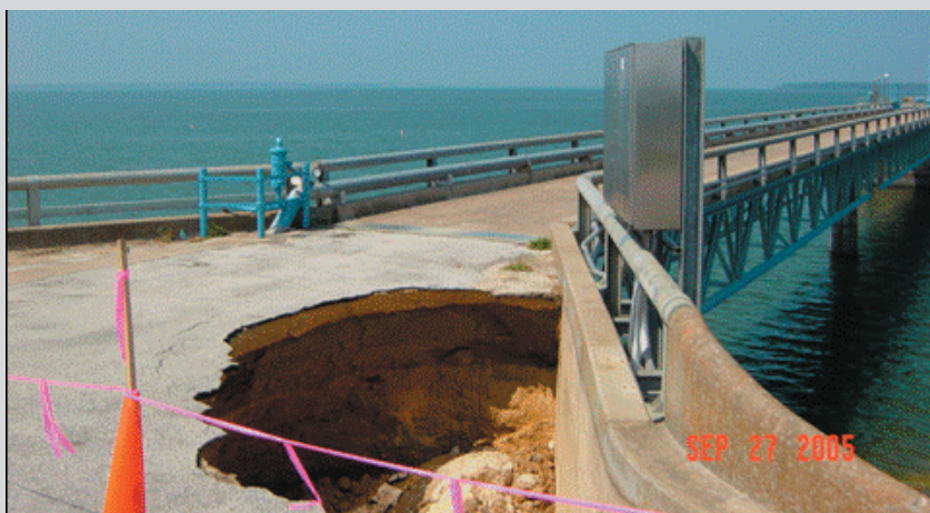
Figure 2. Damage at the Lake Livingston Dam caused by wave action.
