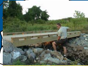
Green Bay FRO Biologist Stewart Cogswell inspects a recently installed bridge that replaced an old culvert. The culvert restricted fish passage along four miles of Sucker Brook. The project was funded in part by the Partners for Fish and Wildlife Program.
