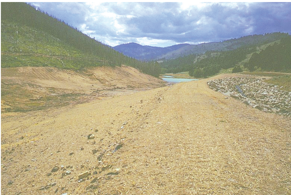
Figure 4. High Ore Creek valley at Comet mine site after remediation activities, August 1998. The creek has been redirected and the area regraded. Photograph by D.A. Nimick.
