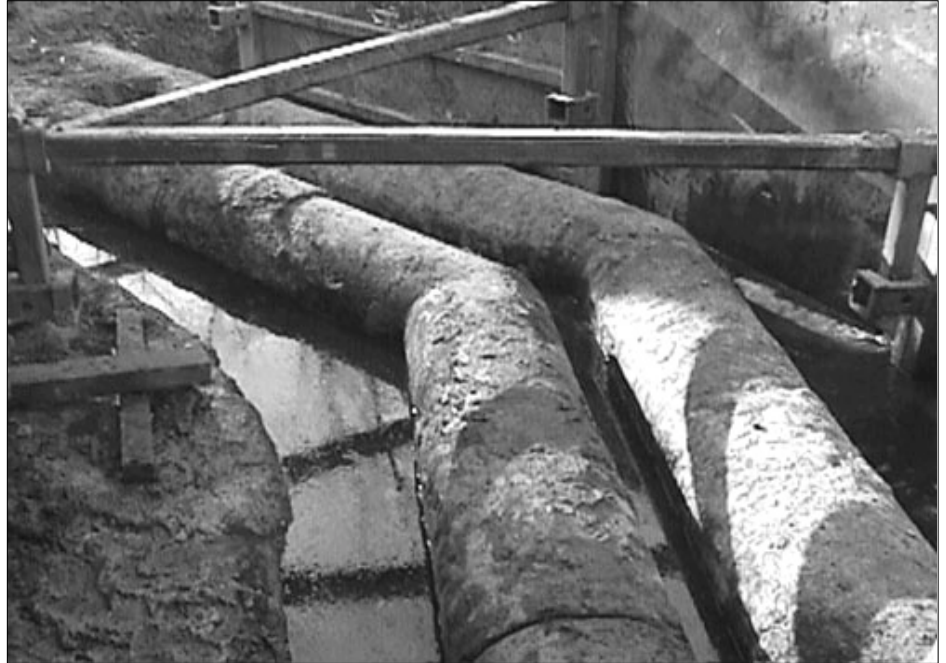
Corrosive pipes can severe environmental damage to the environment that may take years to clean up. (U.S. EPA photograph).
