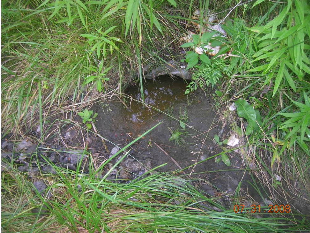
Photo 10 - GE Location 17 - View of the second of two outfall pipes at GE Location 17. This partially silted-in pipe, which is not referenced in Figure 1-2 or Table 3-1, appears to be associated with an adjacent pair of catch basins along Silver Lake Boulevard.
