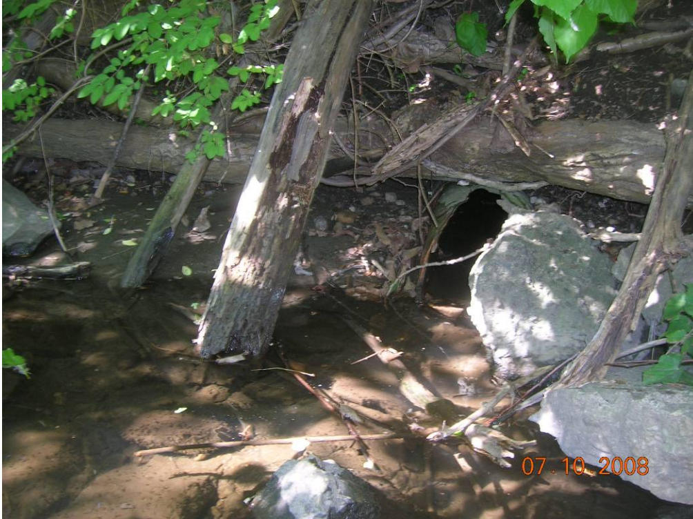
Photo 12 - View of the location of the steel outfall pipe identified by EPA between GE Locations 19 and 20 that is apparently associated with catch basins at the junction of Silver Lake Boulevard and Fourth Street.
