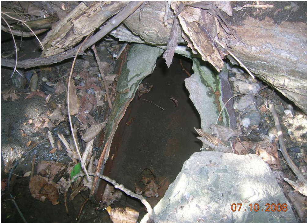
Photo 11 - Close-up view of a steel outfall pipe not identified by GE located between GE Locations 19 and 20 (immediately east of the 42-inch concrete spillway at GE Location 20). This outfall pipe appears to be associated with an adjacent pair of catch basins at the junction of Silver Lake Boulevard and Fourth Street.
