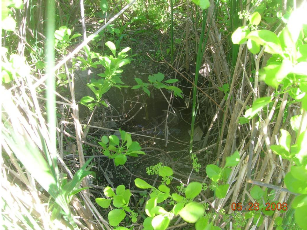
Photo 2 - GE Location 2 - View of the location of the partially silted-in outfall pipe in the vicinity of the “4-inch water blowoff” identified by Hill Engineers in 2006.
