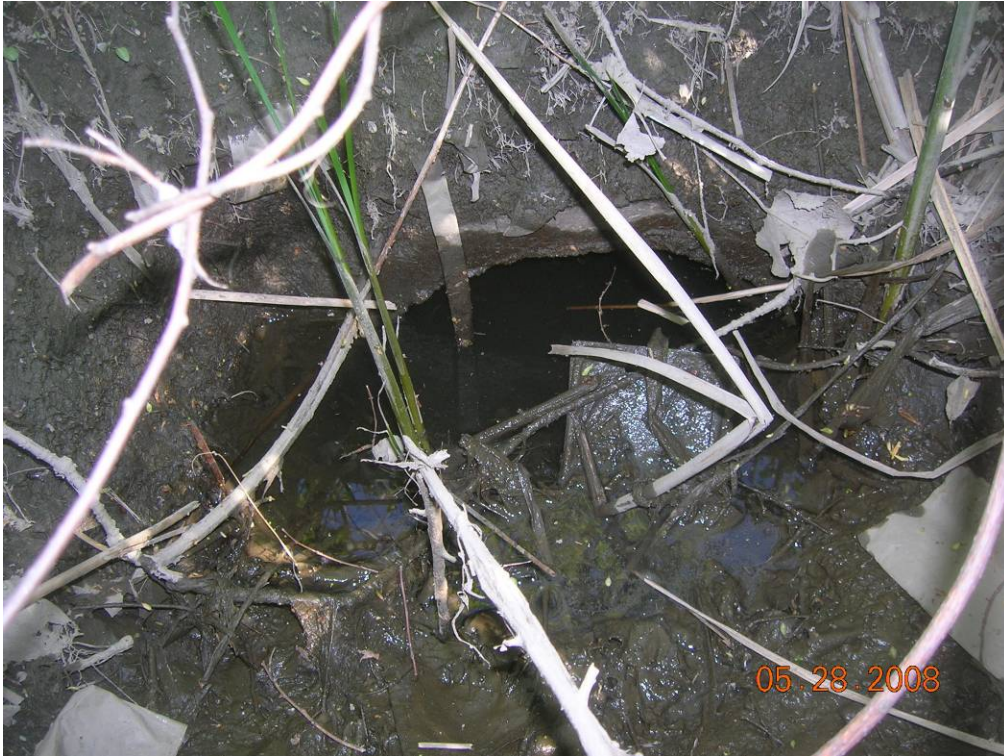
Photo 1 - GE Location 2 - Close-up view of a partially silted-in outfall pipe in the general vicinity of the “4-inch water blowoff” identified by Hill Engineers during September 2006 survey activities, but which GE was unable to locate during its 2008 survey. This location was omitted from Table 3-1 (Outfalls Identified Around Silver Lake) and Figure 1-2 (Silver Lake Site Plan and Existing Conditions) of GE’s July 2008 Conceptual Removal Design/Removal Action Work Plan for Silver Lake Sediments (Conceptual Work Plan) because the pipe could not be located by GE in the field.
