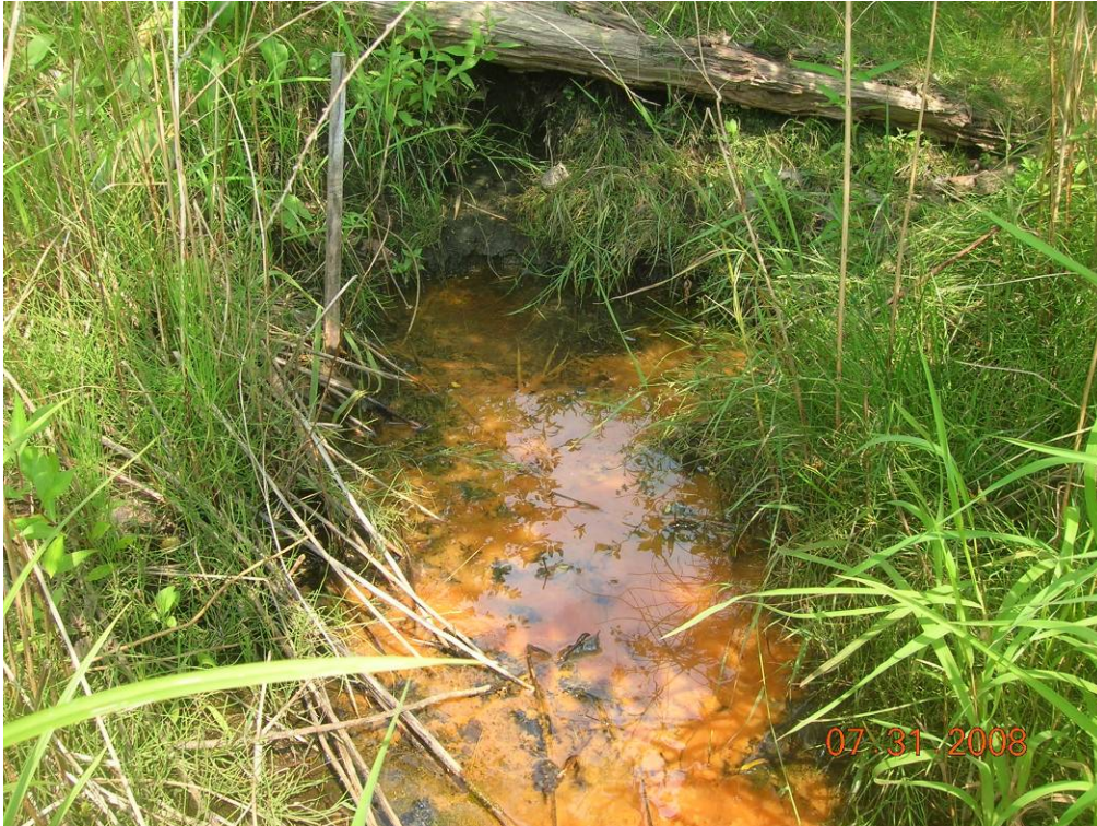
Photo 8 - GE Location 17 - View of the location of one of two outfall pipes at GE Location 17, which were identified by Hill Engineers in September 2006, but which GE referred to as “indications of a pipe” on Figure 1-2 and Table 3-1. There is a subsurface steel pipe at this location.
