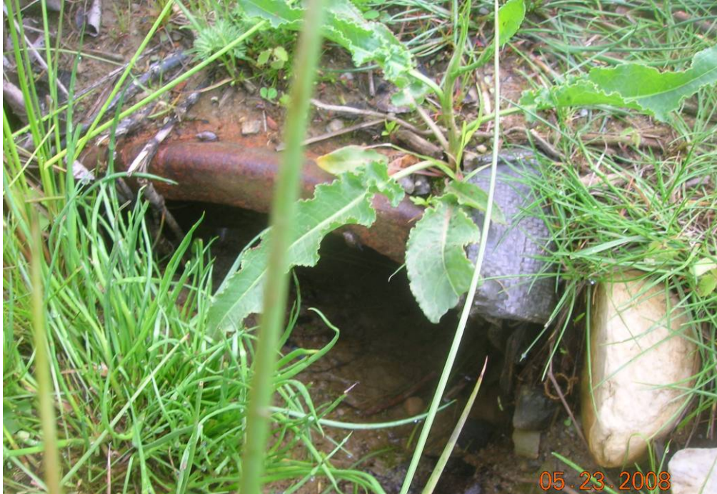
Photo 5 - GE Location 4 - Close-up view of a 20-inch steel outfall pipe at the location EPA believes to be GE NPDES Outfall 004. This location appears to be mapped correctly on GE Figure 1-2, except that GE identifies it as a 12 -inch steel pipe. EPA notes that there is a 12-inch steel pipe approximately 30 feet south of this location that is not presented on Figure 1-2 or Table 3-1. GE appears to be confusing the 20-inch pipe shown above with the 12-inch steel pipe.
