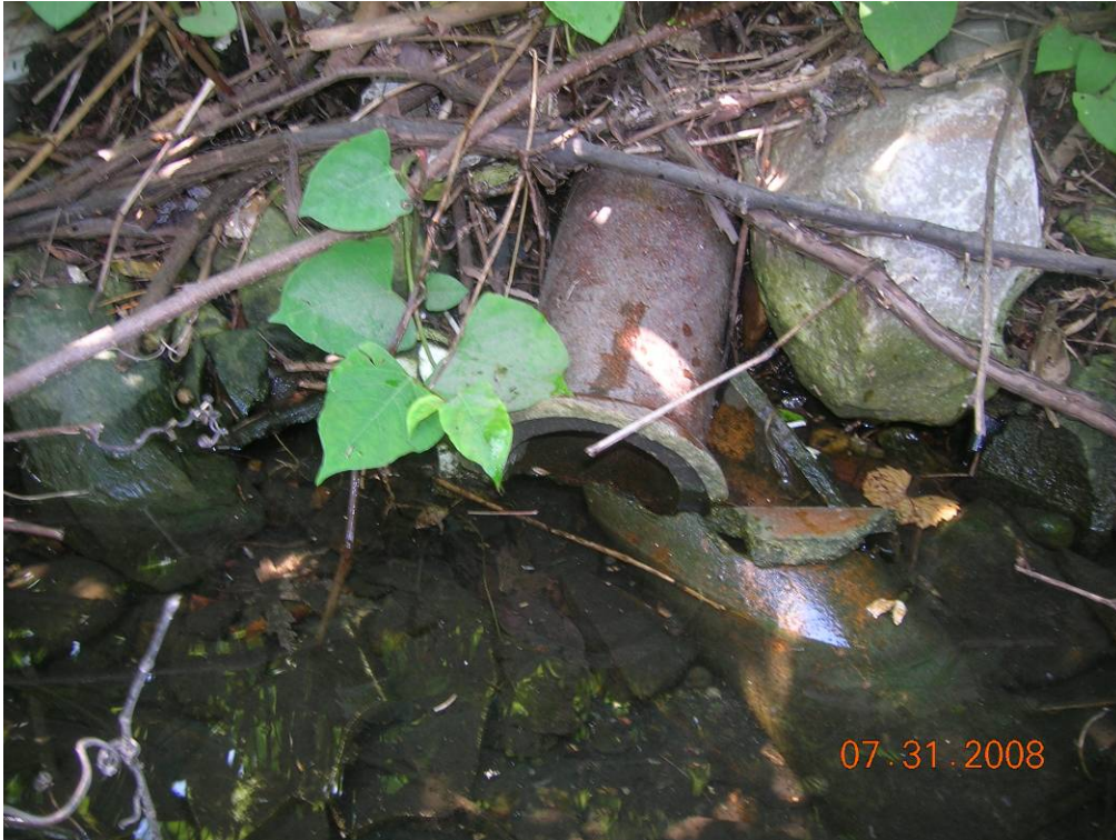
Photo 14 - Close-up view of a clay pipe which was not identified by GE, located between GE Locations 22 and 1, at Parcel I9-9-19.
