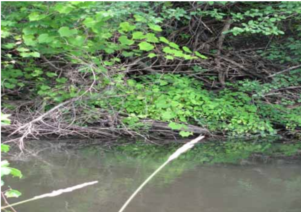
Figure F-11f. Beaver dam and extensive vegetation at downstream end of railroad culvert.
