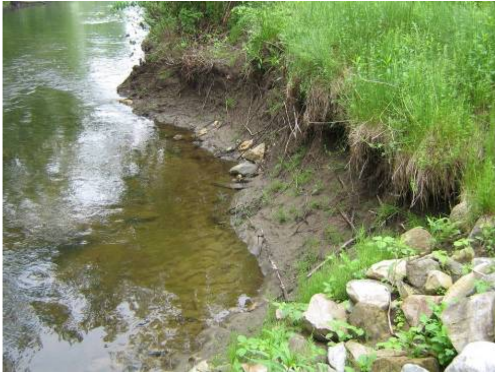
Photo 1 – Area 1: Approximately 25 feet of undercut bank at the end of a section of rip-rap.
