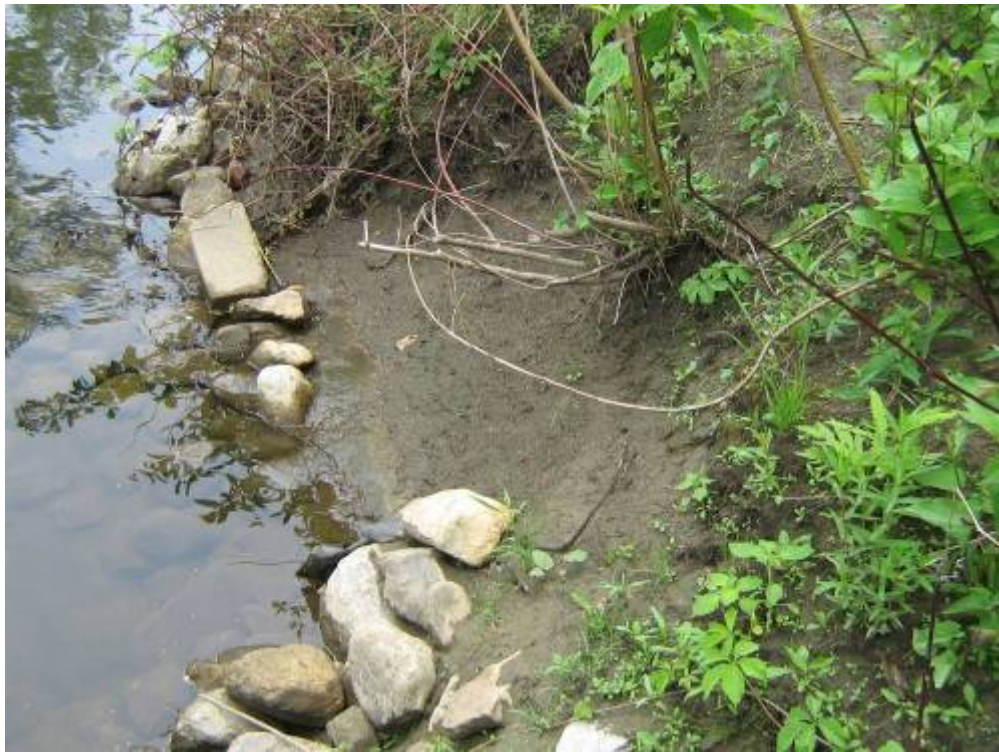
Photo 4 – Area 3: Slight undercut above rip-rap.
