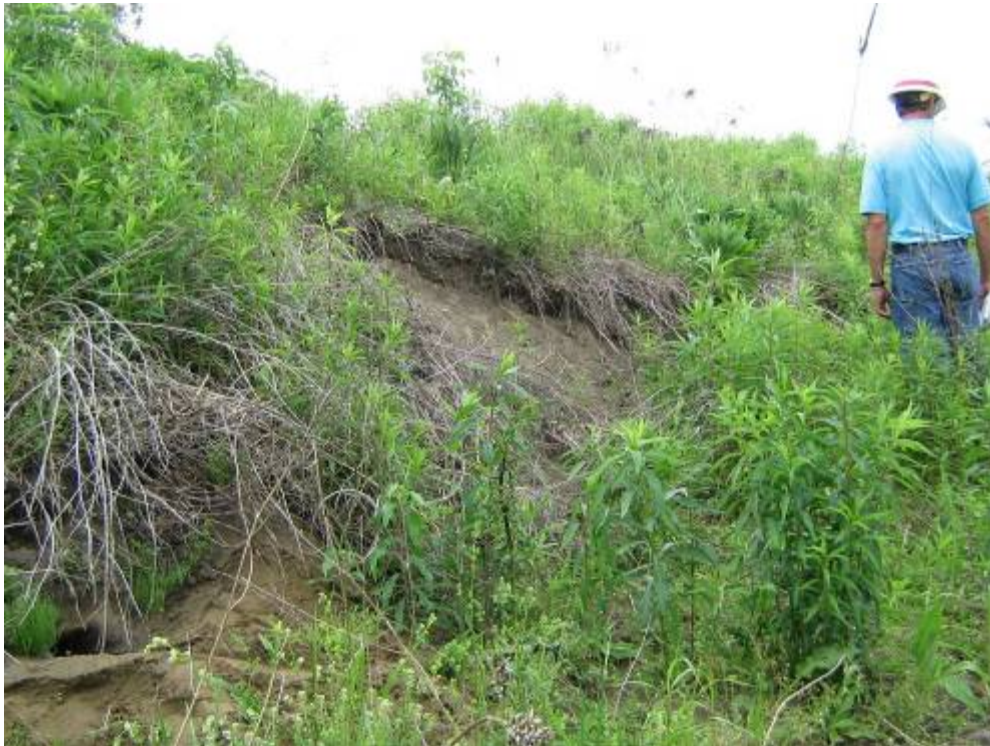
Photo 9 – Area 6: Bank sloughing, no erosion evident.
