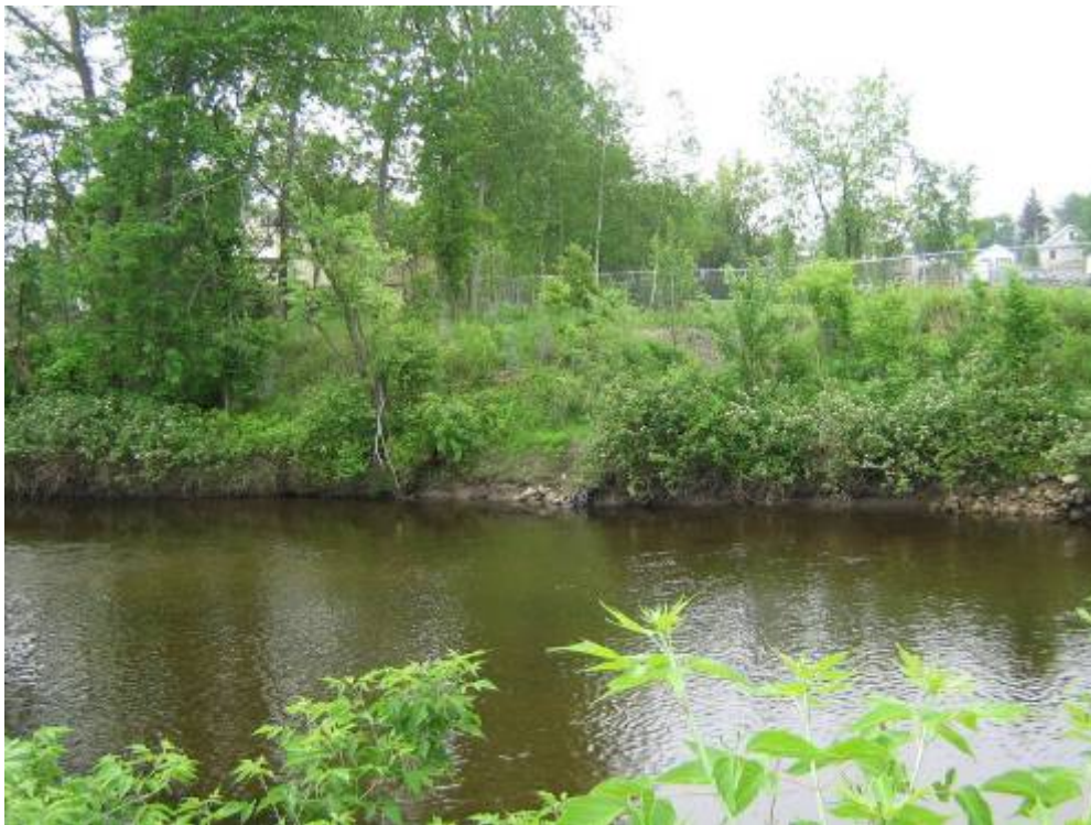
Photo 6 – Area 5: Several small areas undercut above rip-rap.
