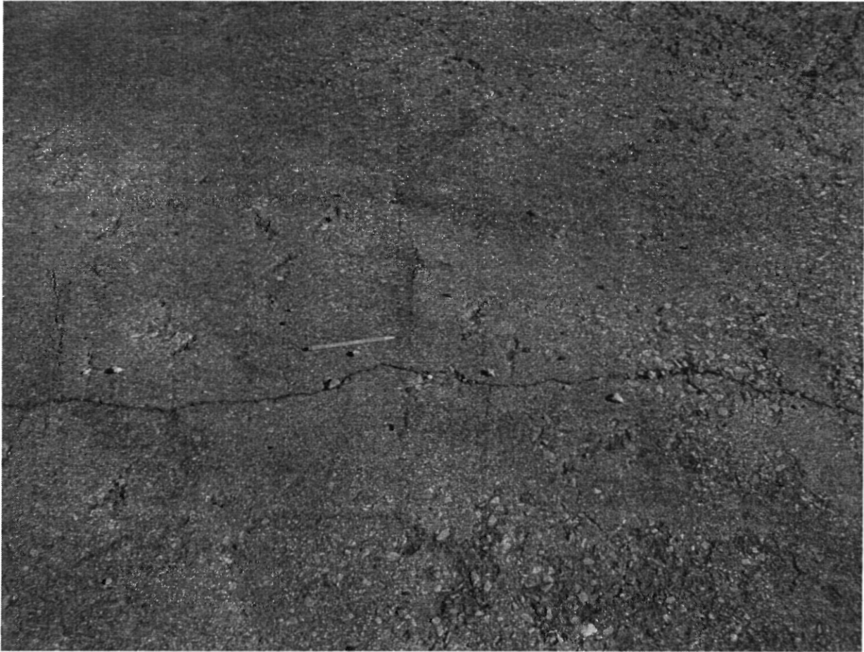
One-quarter to one-half inch crack traversing the approximate center of the barrier November 21, 2008
