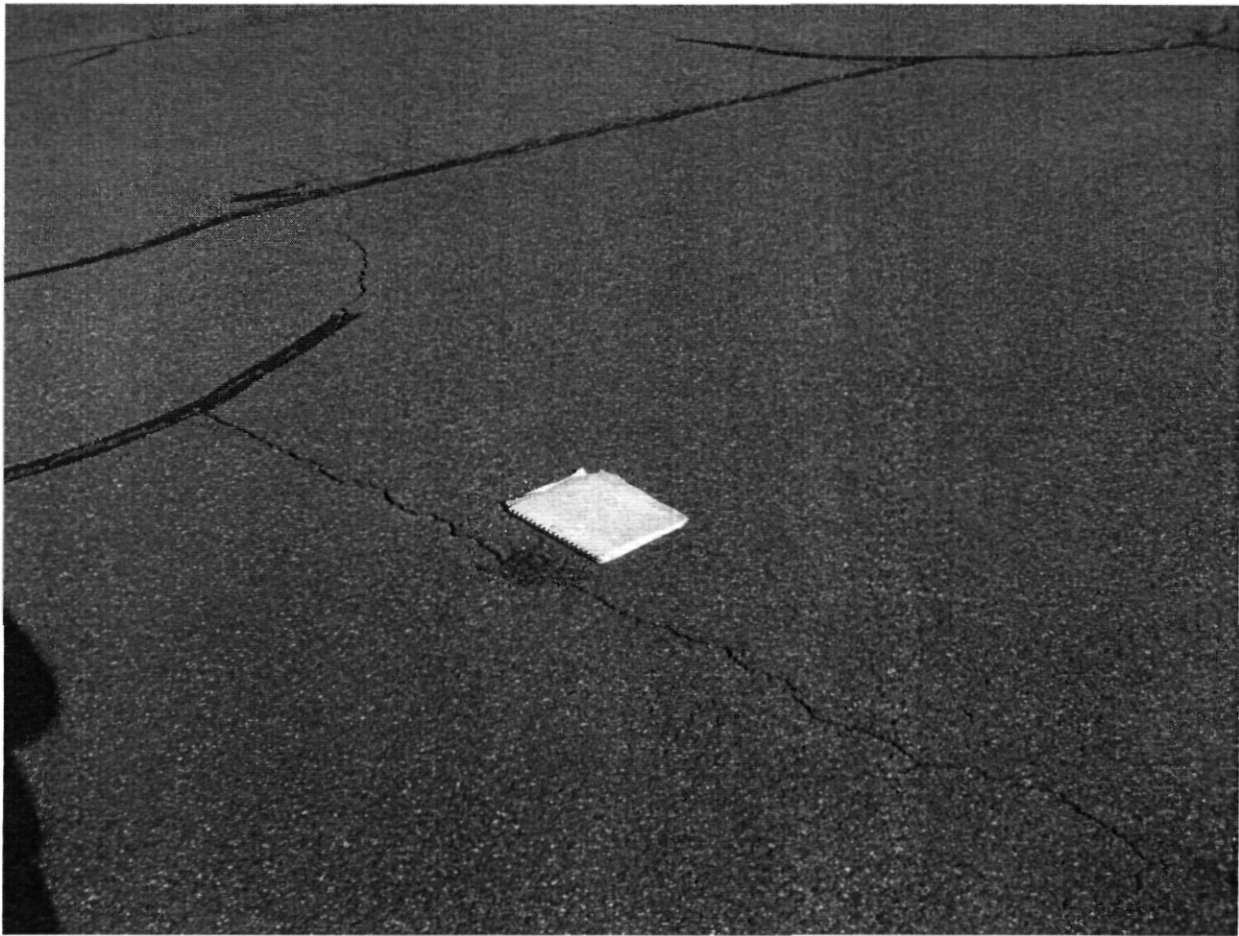
One-quarter inch to one inch crack in the northeastern portion of barrier area November 21, 2008
