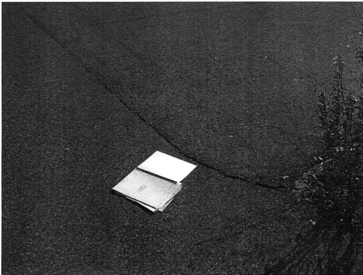
One-quarter to three-quarter inch crack at the northwest edge of the barrier November 21, 2008
