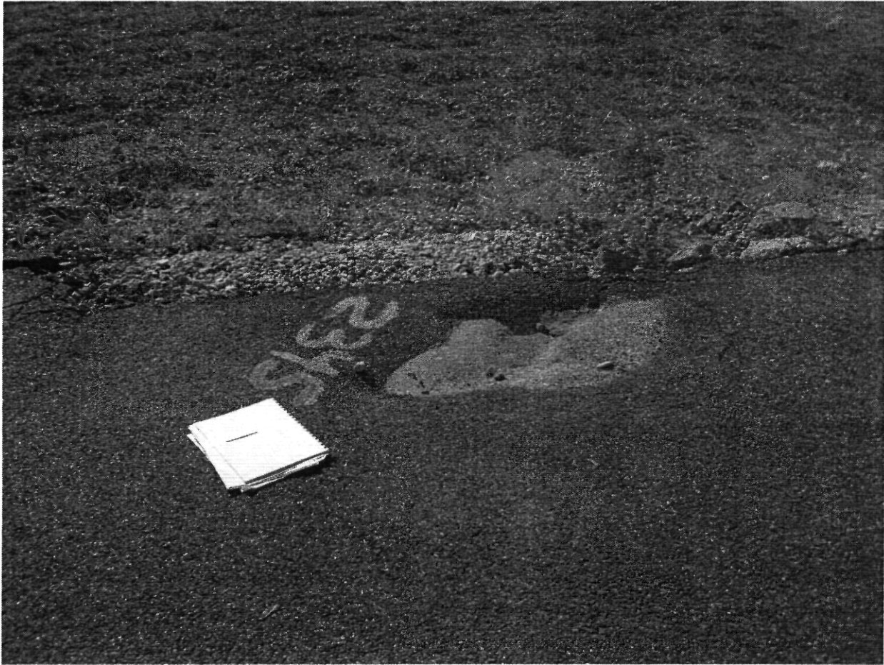
View of depression covered with dirt along southern border of the barrier area November 21, 2008
