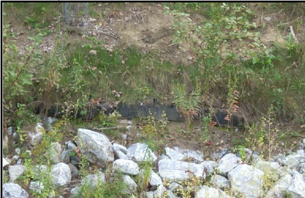
Photograph 10: Area 3C: Exposed Geoweb on Parcel I6-1-68
