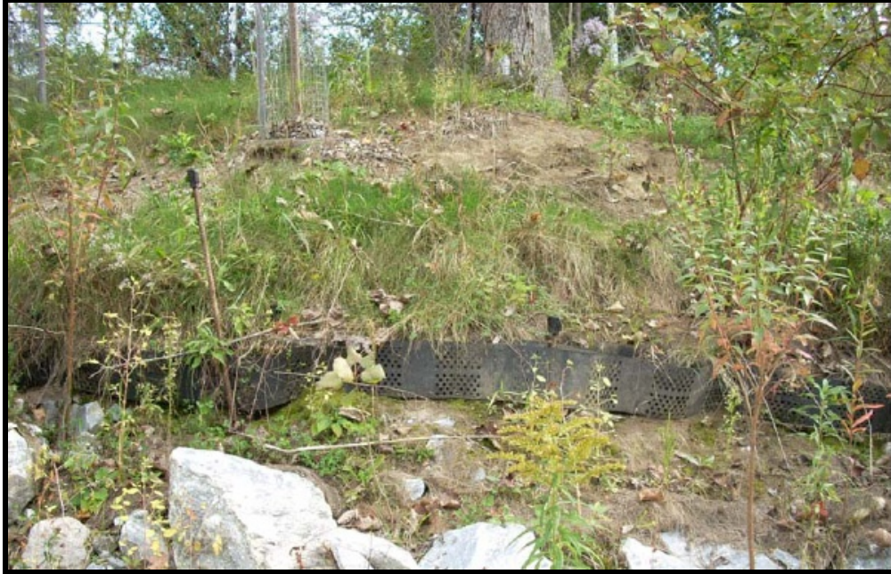
Photograph 9: Area 3C: Exposed Geoweb on Parcel I6-1-68
