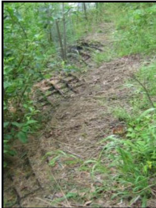
Photograph 6: Area 3A: Exposed Geoweb on Parcel I8-23-6
