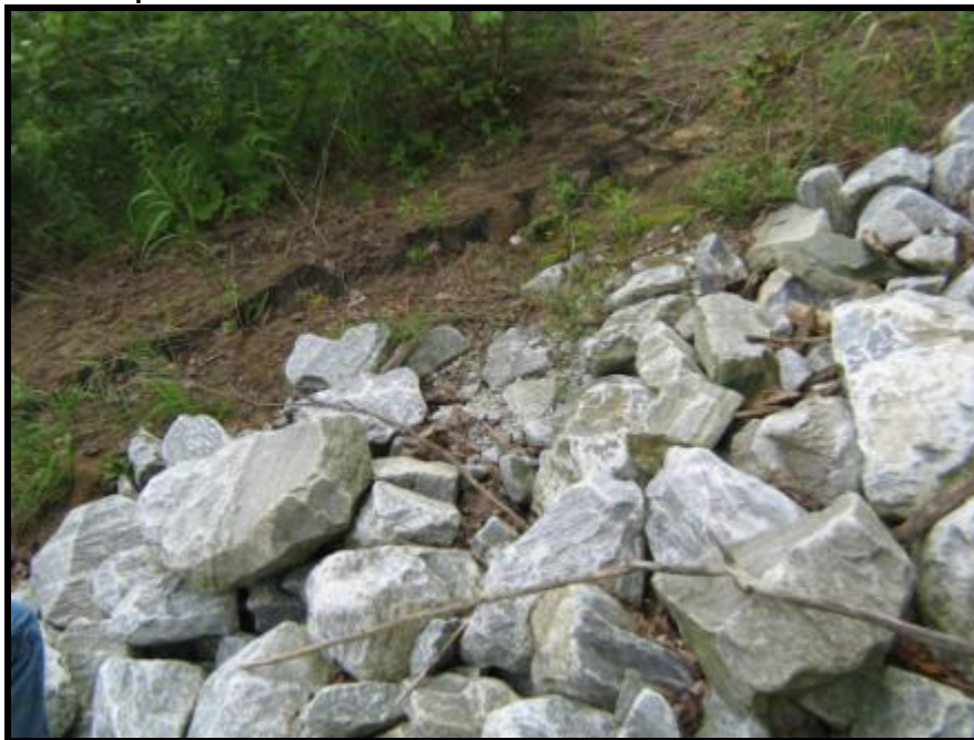
Photograph 8: Area 3B: Exposed Geoweb on Parcel I8-23-2/3
