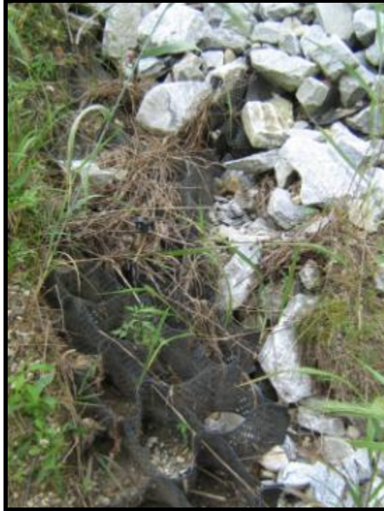
Photograph 5: Area 3A: Exposed Geoweb on Parcel I8-23-4
