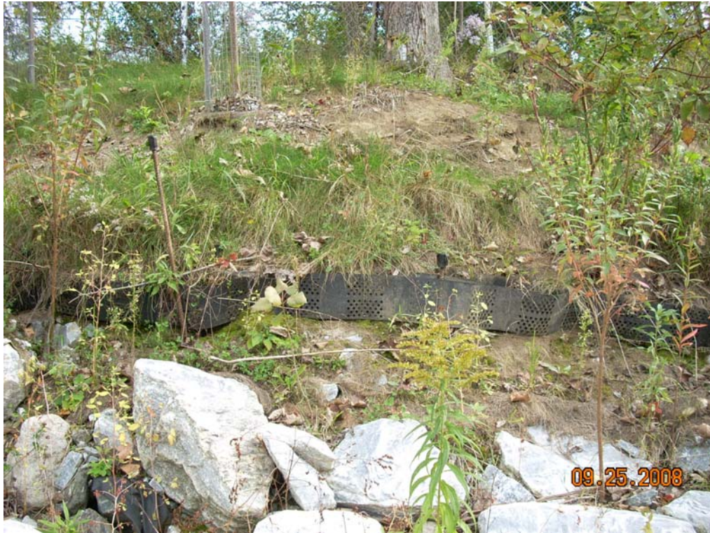
Photographs of Erosion above the riprap on Parcel I6-1-68 that requires stabilization
