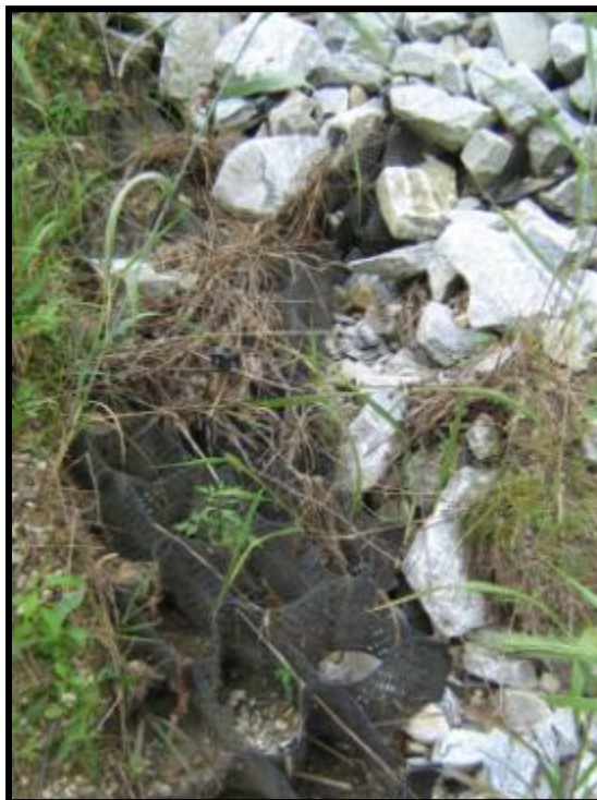
Photograph 6: Area 3: Exposed Geoweb on Parcel I8-23-4
