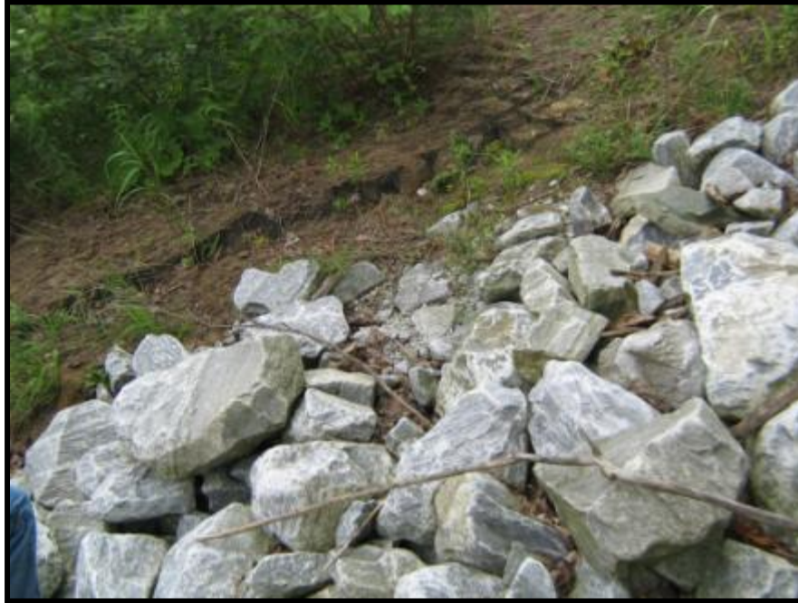
Photograph 5: Area 3: Exposed Geoweb upstream of Swale near Parcel I8-23-4
