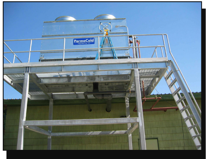
Figure 5—The condenser for the new refrigeration system also provides a warm water source for defrosting the cooler room evaporators at the Coeur d'Alene Nursery.
