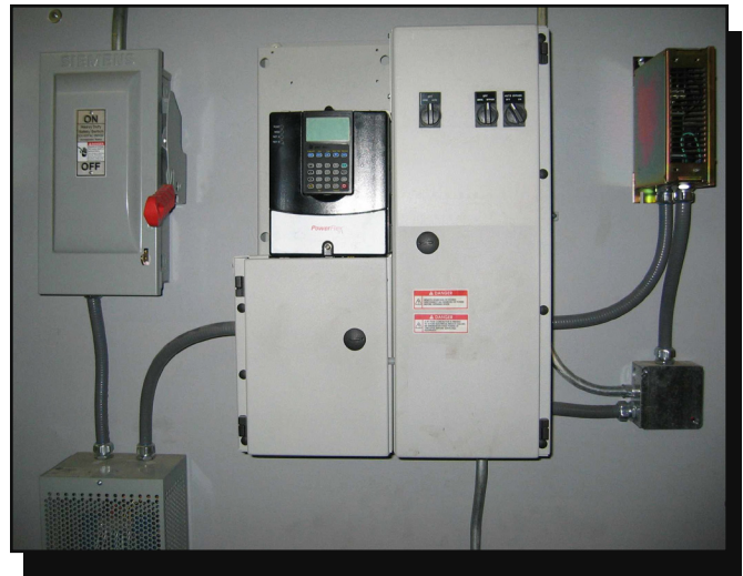
Figure 4—This variable frequency drive controls the speed of the motors on the evaporators inside the cooler rooms at the Coeur d'Alene Nursery.
