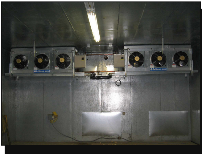
Figure 3—New, efficient evaporators inside each cooler room at the Coeur d'Alene Nursery replaced large, power-hungry evaporators located outside the cooler walls.
