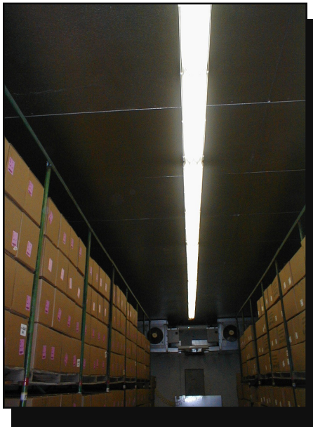
Figure 6—The new light fixtures in this packing shed at the Coeur d'Alene Nursery are far more energy efficient and contain far less toxic material than the old fixtures.
