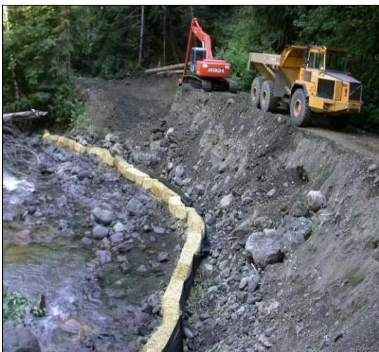
Road repair on Olympic National Forest following damage caused by storms in 2006. (Courtesy U.S. Forest Service)
