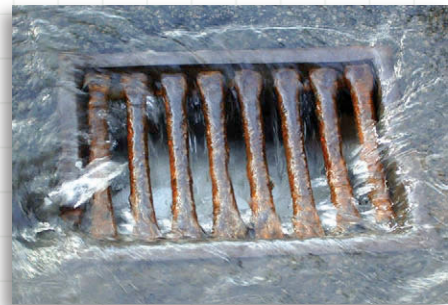
Stormwater runoff from roads, parking lots, and other impervious surfaces flows into storm drains, which lead to nearby waterbodies.
