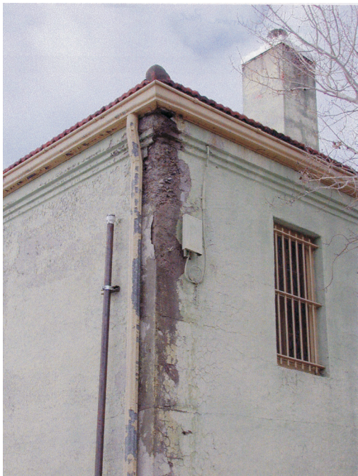
Fort Yellowstone jail is slowly crumbling from lack of maintenance. Water intrusion and subsequent freezing and thawing have caused half of this historic structure to erode.
