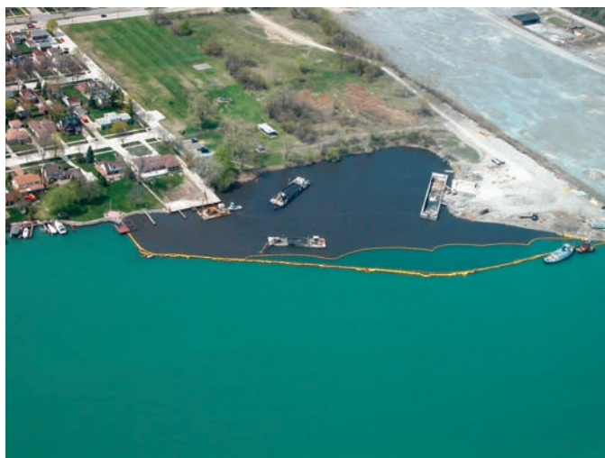
While EPA and the Michigan Department of Environmental Quality dredged the Black Lagoon, yellow silt barriers kept contaminated sediments from spreading in the Detroit River.
