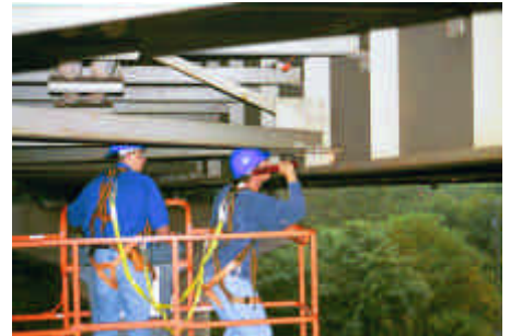
An inspector looks for defects in the superstructure of a bridge in Virginia.
