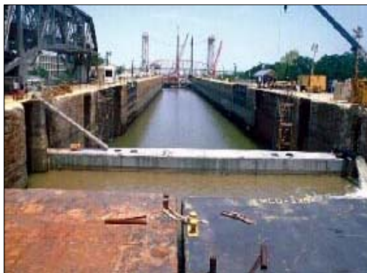
De-watering and repairs of the Inner Harbor Navigation Canal Lock, New Orleans.
