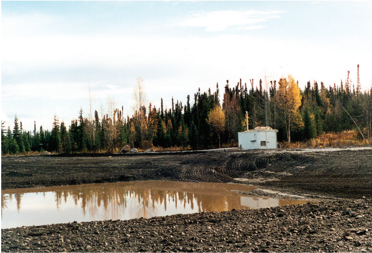
Incomplete engineered wetland at the Pipe and Supply Yard at Swanson River Field. USFWS Photo by Tiffany A. S. Parson.
