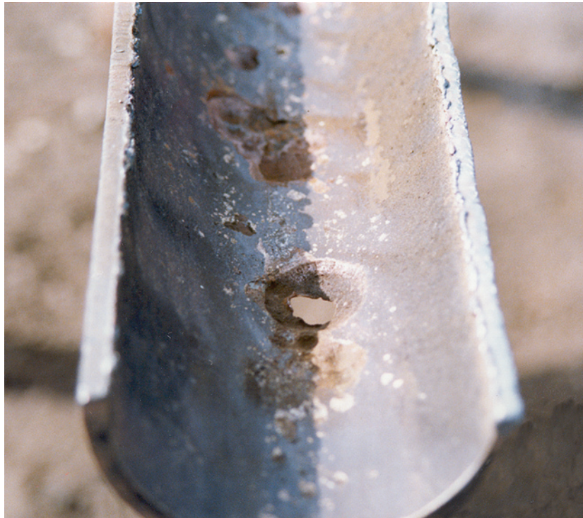
Severe corrosion in the 2-15 drain line prompted an extensive effort to determine the integrity characteristics of other long-buried lines within Swanson River Field. USFWS Photo by James E. Frates.
