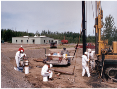
A site assessment of each flare stack delineated the extent of crude contamination. USFWS Photo by Robert A. Richey.
