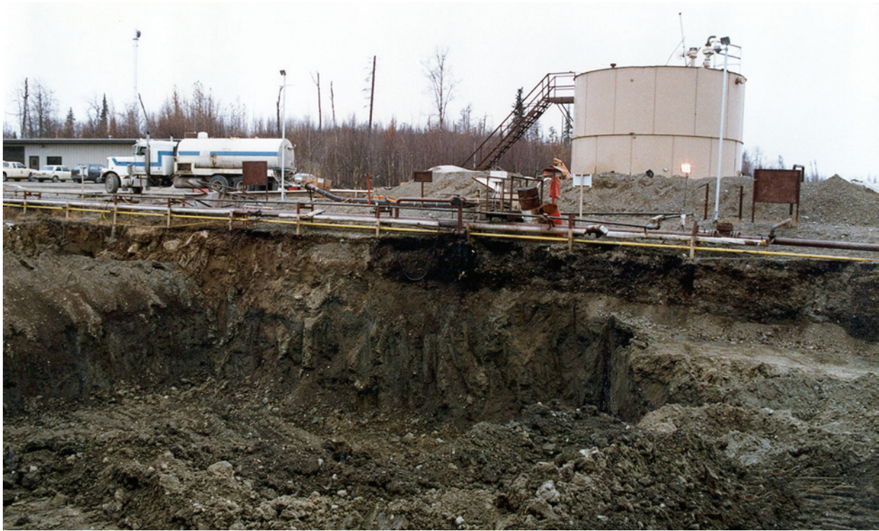
Excavation of contaminated soils resulting from the tank farm spill. USFWS Photo by Robert A. Richey.
