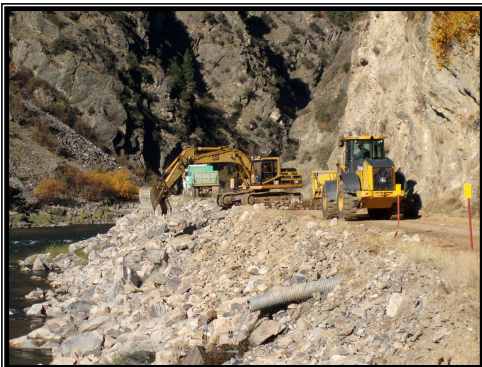
Main Salmon River Road Repairs and Maintenance preparation for dust palliative application.
