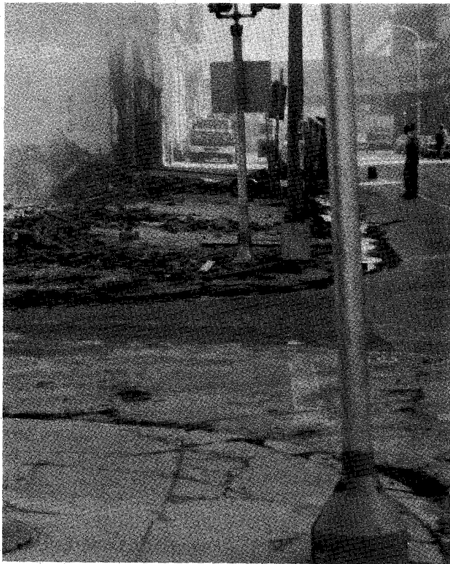
Figure 24. Building demolition without pedestrian protection
