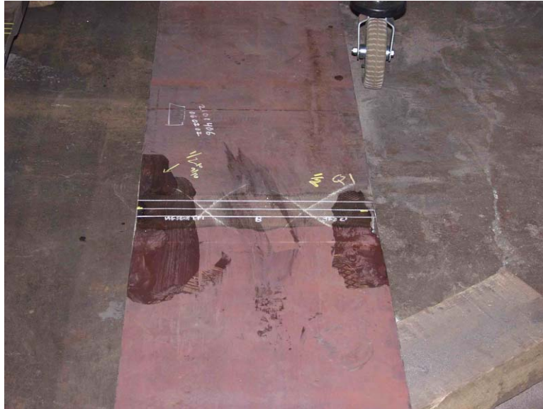
Figure 83. Field specimen G5G-TF1-TopF: Top view of joint.
