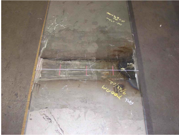
Figure 113. Field specimen FG37K-TF3-BottF-FCM: Top view of joint.
