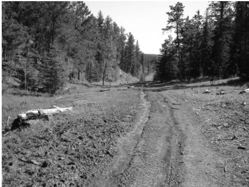
Figure 5. A maintenance level 2 road with damage caused by ATV track following. The damage is increased by erosion when the tracks channel water down the road.
