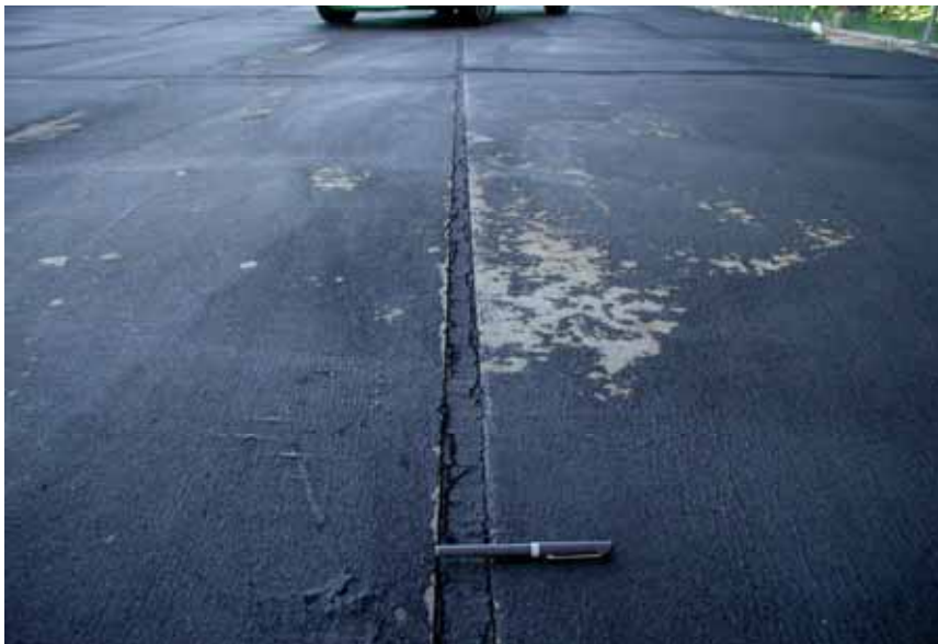
Figure 2-14. Heaving of a slab relative to another
