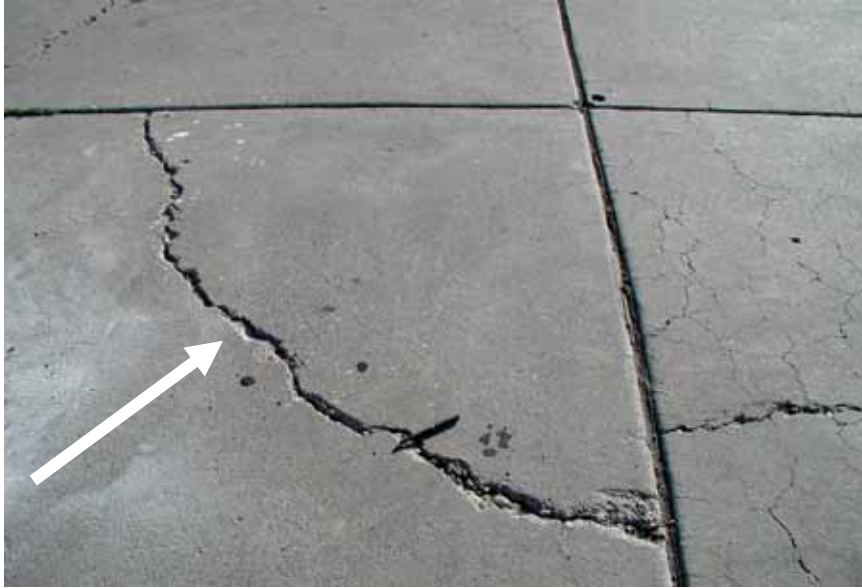
Figure 2-16. Corner break (→) in an airfield pavement.
