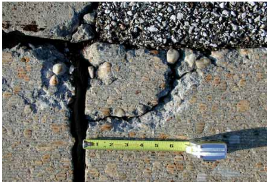
Figure 2-17. Corner spall in another airfield pavement.
