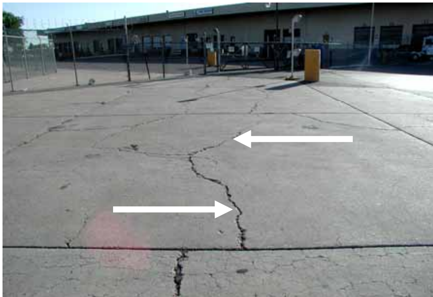
Figure 2-19. Longitudinal cracks (→) in an airfield pavement.
