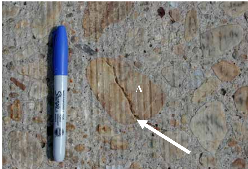
Figure 2-8. An open internal crack (→) in an ASR-affected aggregate particle (A).
