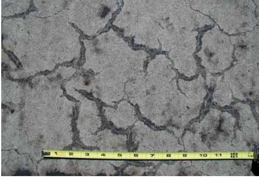
Figure 2-9. Gel exudation through cracks.
