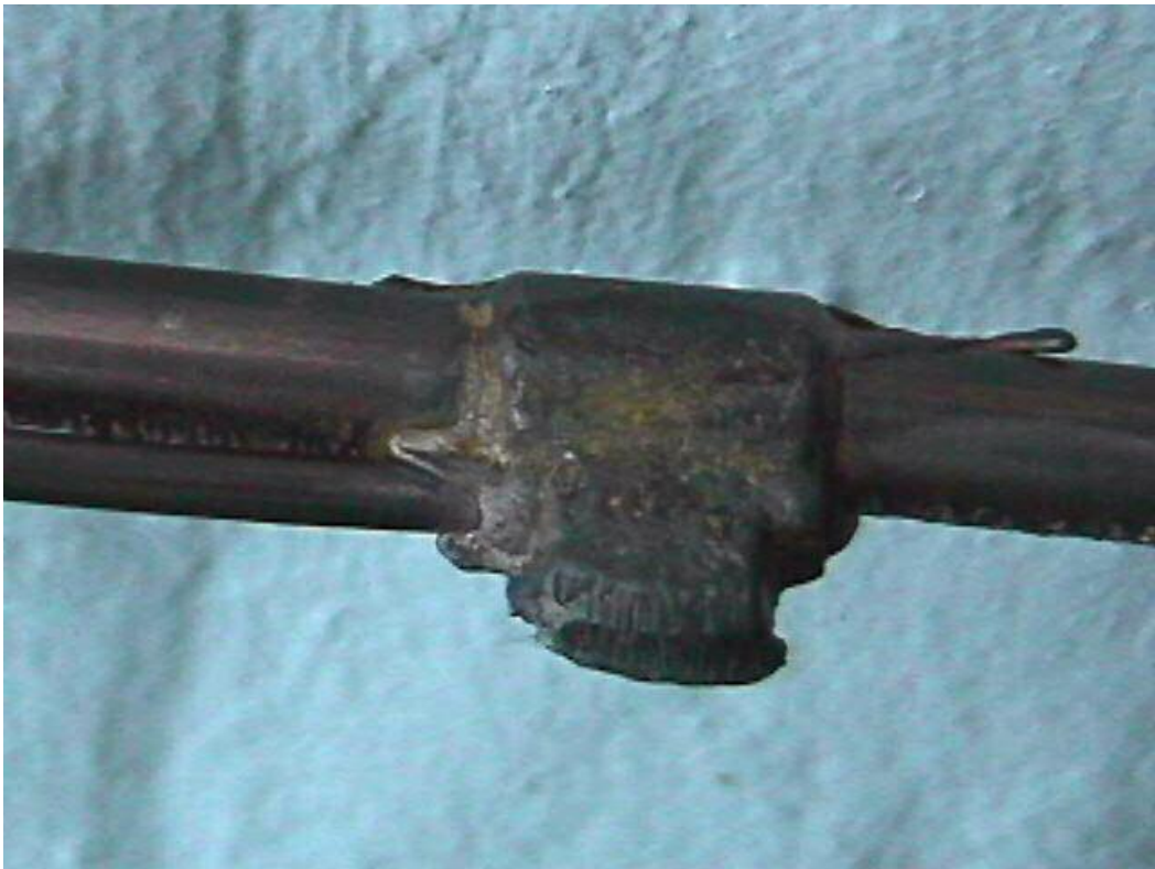
No. 4 : We can clearly see the above mentioned welding.
