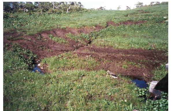
Without careful use, motor vehicles can damage the land. Damage to meadow from cross-country use, Harbor Mountain Trail, Tongass National Forest, Alaska.
