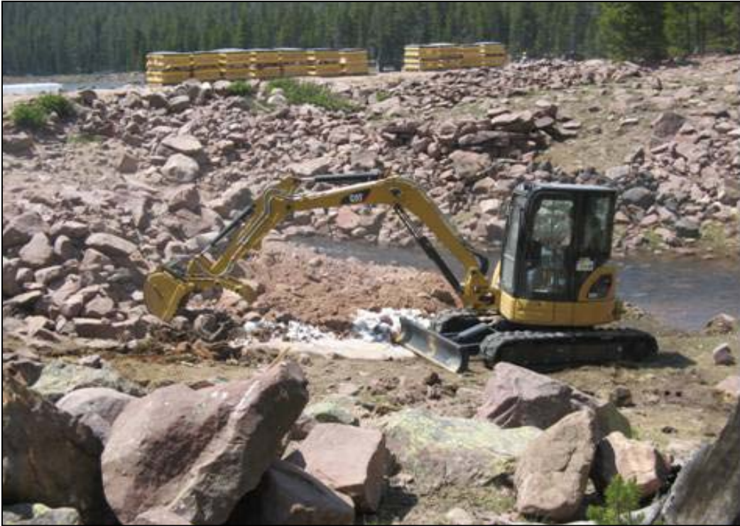
Small excavator removes material from the dam at Brown Duck Lake in the high Uintas wilderness
