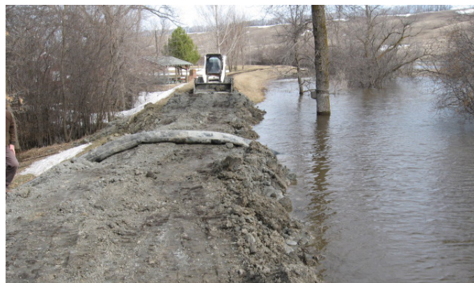
FWS personnel work to strengthen dikes at Valley City NFH and WMD Headquarters, Valley City, ND Chad Zorn / USFWS
