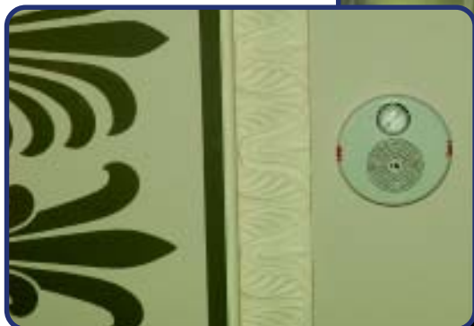
Fire alarm inconspicuously placed in ceiling. The stenciling was repainted during the modernization process.
