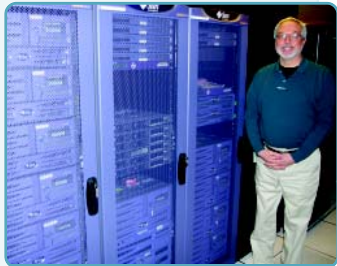
Fred Schneider, UNIX Technical Lead who works for the Denver office of NBC, stands next to some of the servers that have been installed to support FBMS production activities.
