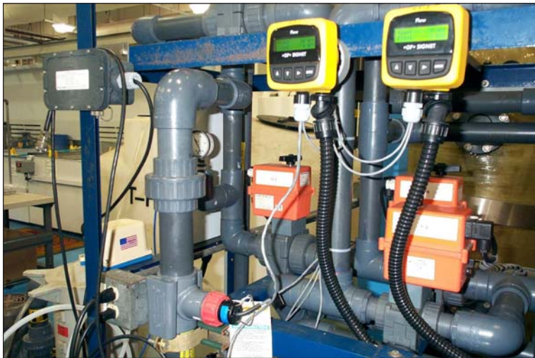
Photo 5. Signet flow totalizers and flow sensor (bottom).
