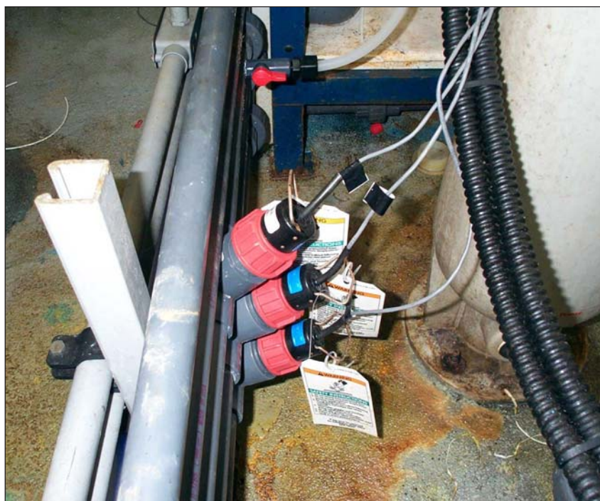
Photo 6. Flow sensors installed in feed lines. Valve and sampling line for regenerant waste is shown at rear.
