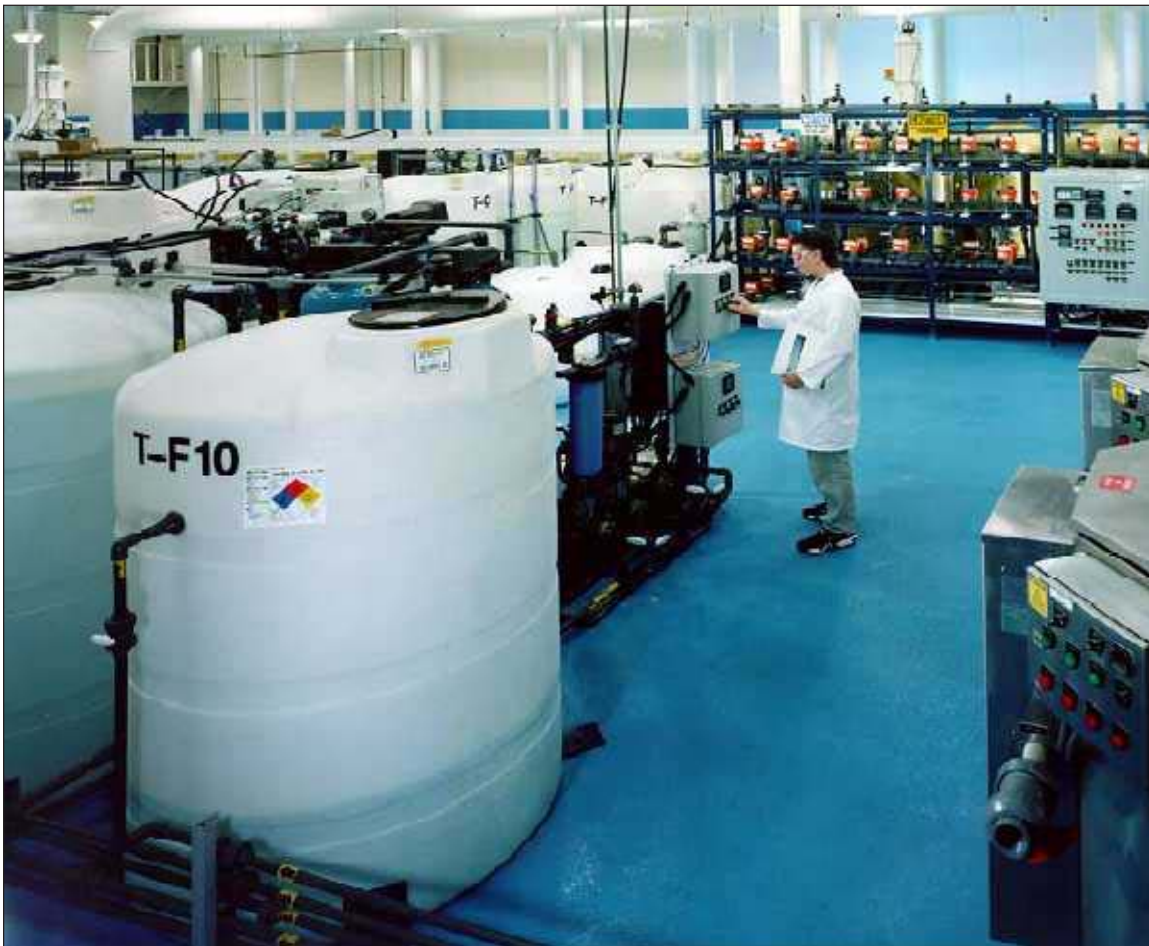
Photo 1. Aero-Electric Connector, Inc. facilities in Torrance, California, showing installation of Hydromatix 786E Ion Exchange treatment system and associated equipment.
