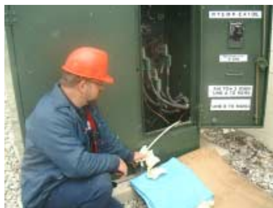
Figure 5. Transformer Sampling at Cooper
