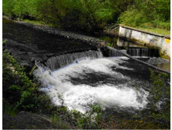
Before project photo of Kooskooskie Dam, a barrier to migrating salmon on Mill Creek. Photo: Washington Department of Fish and Wildlife - LIP Program
