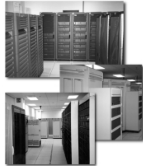
The OIG conducted vulnerability tests of servers at Postal Service Headquarters and three other locations nationwide.
