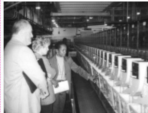
The OIG evaluates vital mail systems including the Automated Flat Sorting Machine 100, which automates processing of mail larger than a letter incorporating on-site barcode technology.
